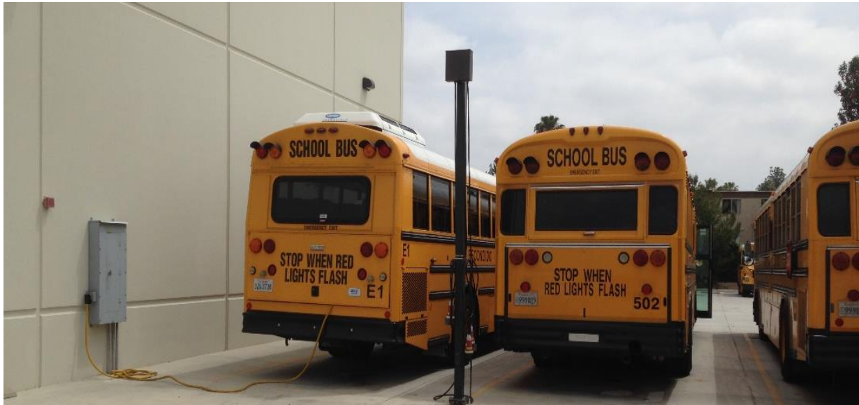
Figure 18. EESB Plugged In at CVUSD using same 208VAC panel as used for DPFs
