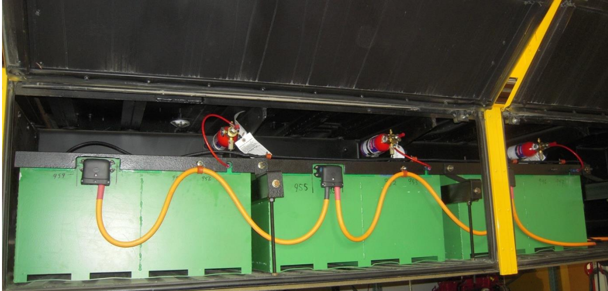
Figure 9. Battery modules mounted in one side of EESB prototype luggage compartment.
