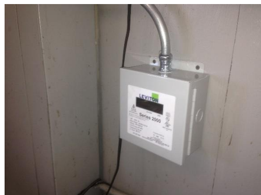
Figure 19. EUHSD kWh meter
