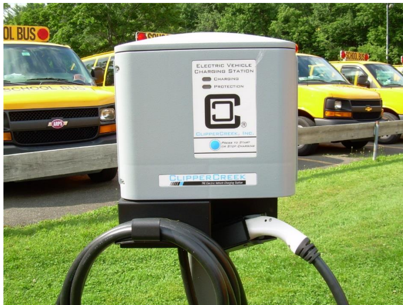
Amherst Clipper Creek Electric School Bus Charging Unit.
