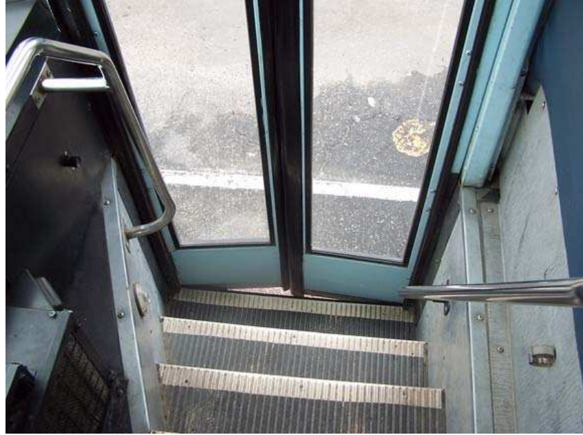
Photograph 3.2.2.1 A leak at the bottom of a bus door.
